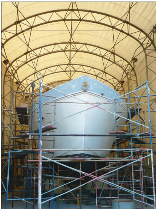
Due to limitations on new buildings built within 100' (30.4m) of the high-water mark, many of KKMI's shelters for larger boats are temporary fabric-covered structures such as this one for a 1970s motor-yacht in for core repairs and a paint job.
